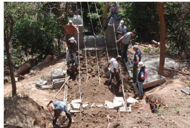
Undergraduate students from the Department of Civil and Environmental Engineering help build a bridge in Nicaragua. The students traveled with the Engineers Without Borders organization of the College of Engineering.
